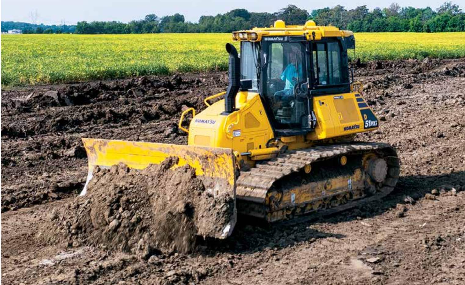
With a Komatsu D51PXi-24 IMC dozer, an operator cuts material to grade for a new access road.
