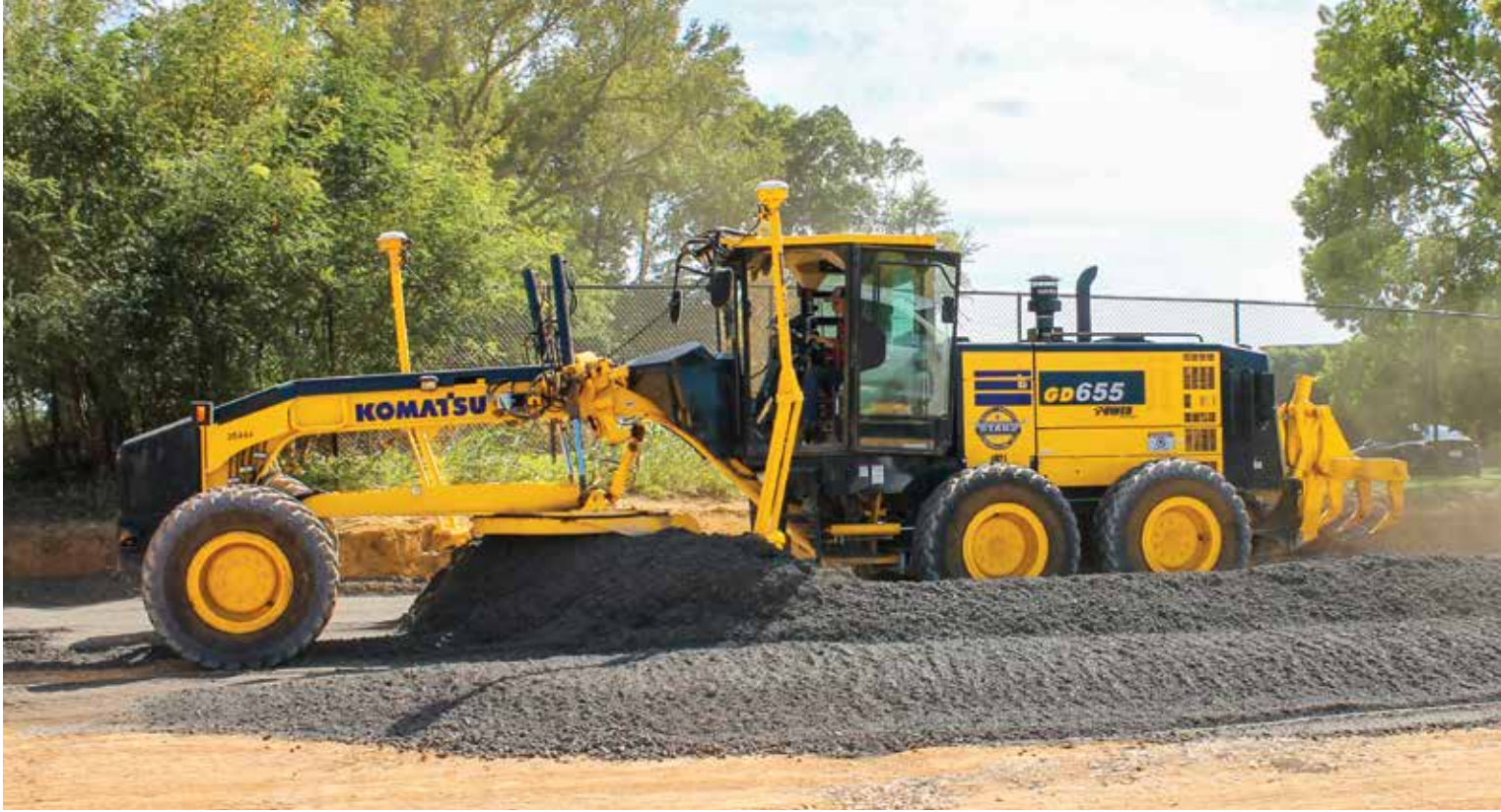
The Komatsu GD655 motor grader helps Byard Construction reach grade with precision.
