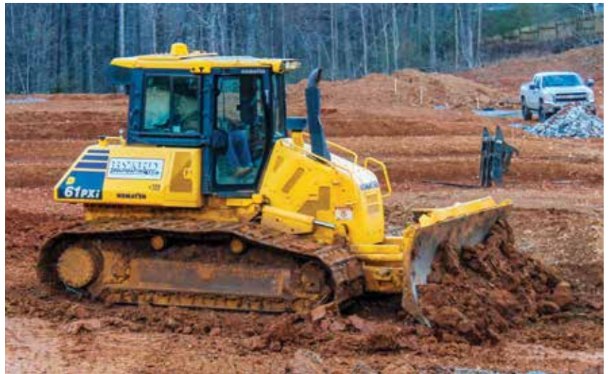
Using a Komatsu D61PXi IMC dozer, an operator cuts material to grade.
